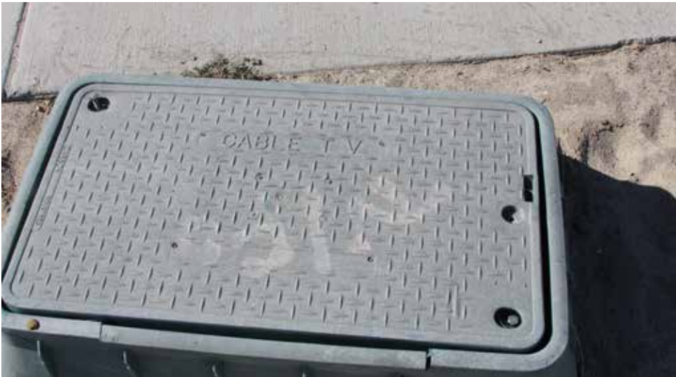
Cable TV Utility Box
